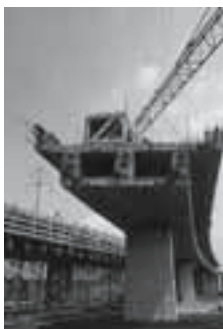
Construction of the new rail line from Zurich to Kloten. Motor-Columbus planned, designed and managed the underground works for the Oerlikon-Glattbrugg section.
