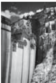
Construction of the El Cajon dam in Honduras, 1979–1985. Project planned by Motor-Columbus Ingenieurunternehmung.
